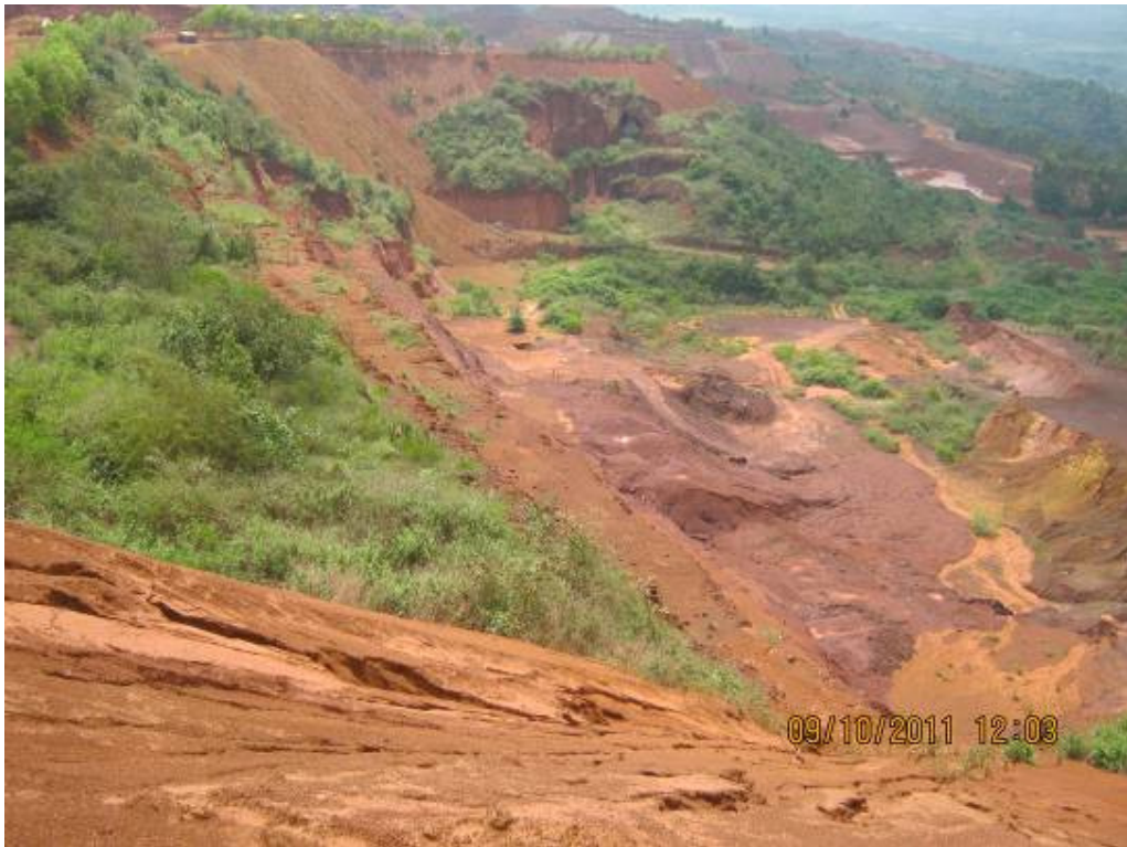
Flowing of silt towards natural nala from unstabilized steep OB dumps of Ganapathi mines of Tumkur
