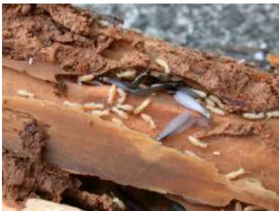
Termite attack on wood
