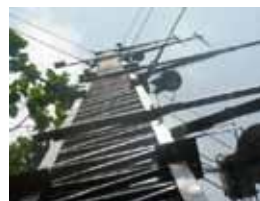
Betul Tower, Sensors shown on different levels
